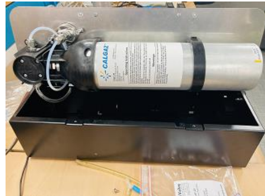
Connected gas cylinder.
